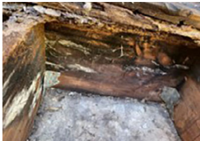
Figure 13. Example of insufficient or no waterproofing affecting a balustrade on a funded building in CSV's program (comprising 12 sole occupancy units)
