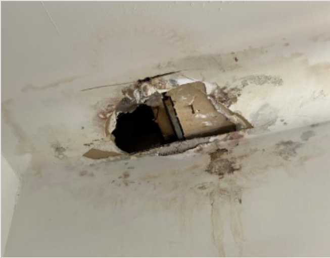
Mould and staining on apartment ceiling.
