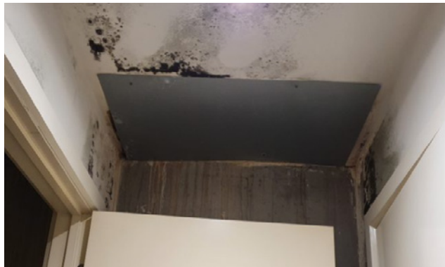
Figure 8. Black mould on the ceiling and walls in this apartment
