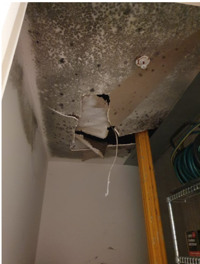
Figure 7. This apartment's ceiling has collapsed after years of water collected from the balcony above it
