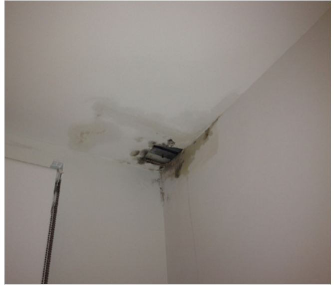
Moisture seeping through plaster walls.
