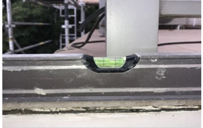
Balcony falling steeply away at edge.
