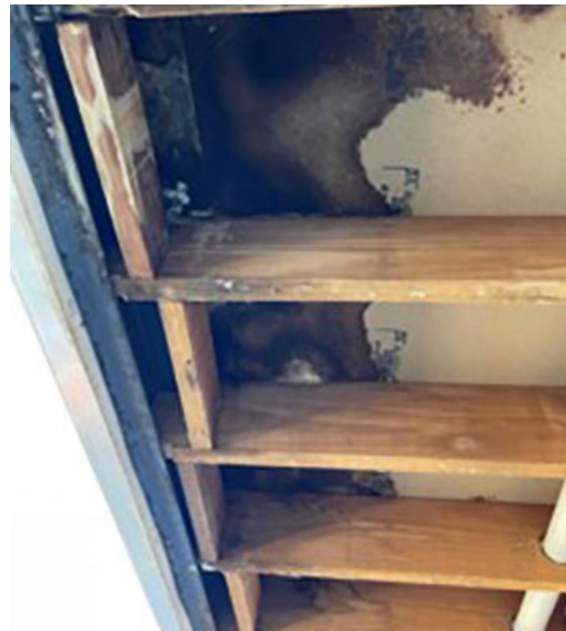
Underside of balcony; substrate with significant rot from water and timber joists showing rot.
