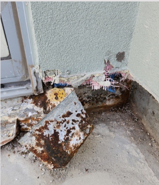
Corroded steel frames caused by water leakage.
