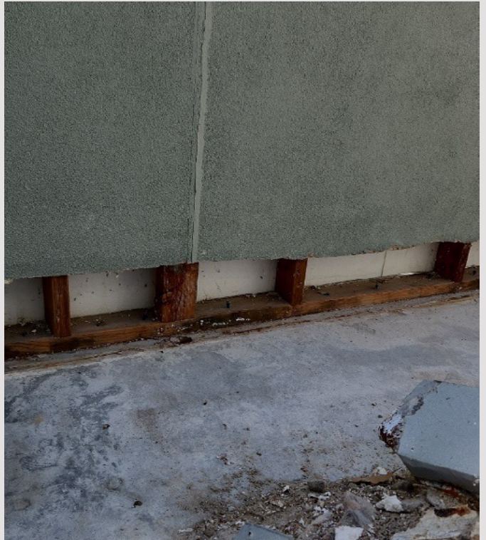
Example of waterproofing damage that is being replaced.
