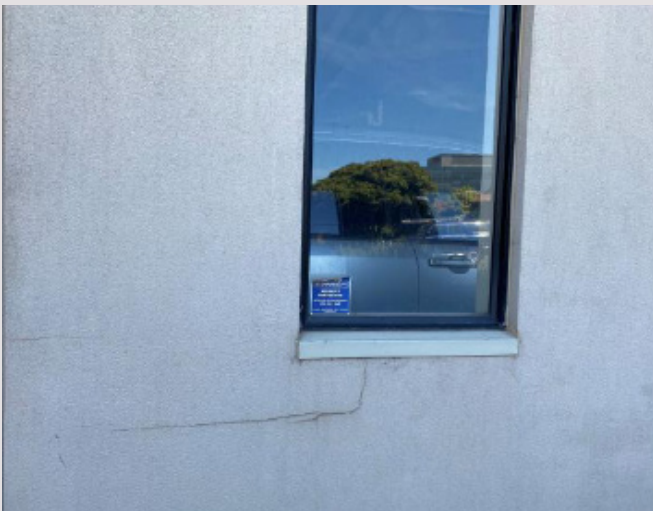
Cracking along blockwork joints.
