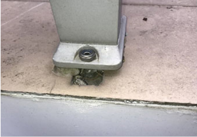
Improper water proofing around balustrade fixing providing areas for water ingress to structural elements.
