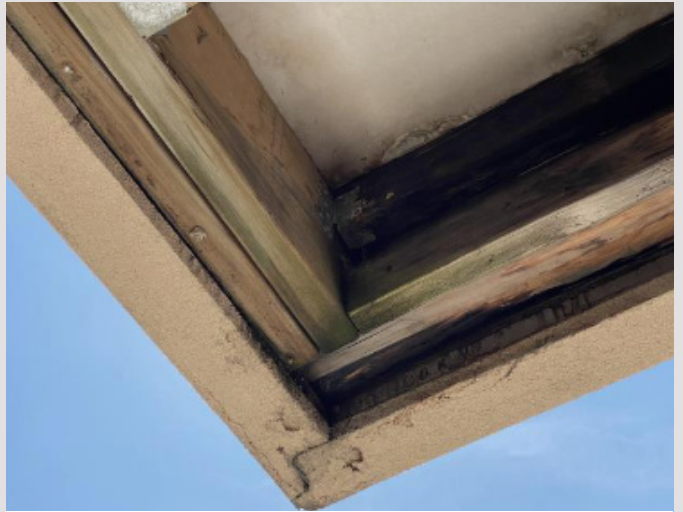
Deterioration of timber balcony.
