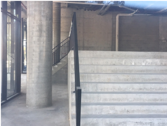
Figure 5: Gravity Tower ground floor tenancy (from Montague Street) with internal stairs to approximately 1.7-1.8m in height.
