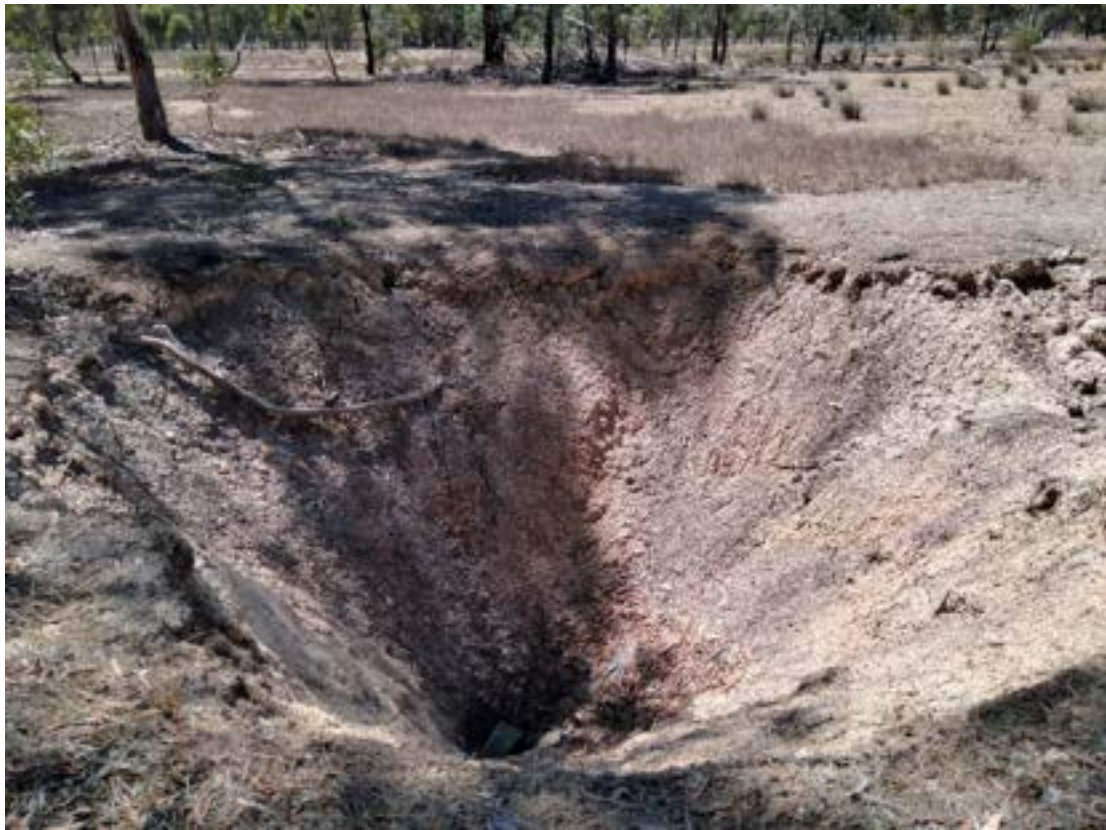
Collapsing mineshaft - February 2022
