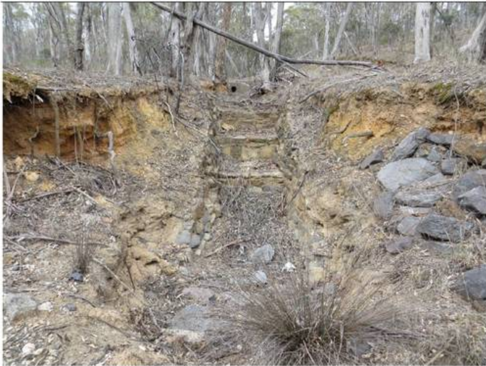
Field stone and mortar stepped water flow feature (HF005) in water race/channel HF001.
