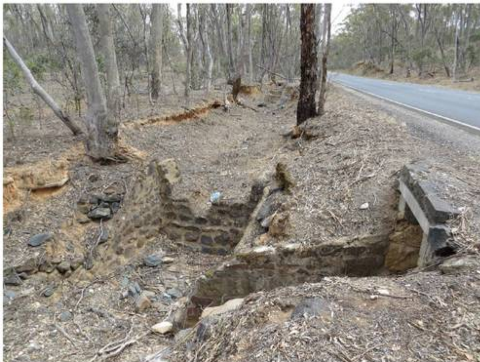
Field stone and mortar hydraulic water flow control feature HF003 in situ in water race feature HF001. Roadway sandstone box culvert can be seen at right, built into features HF001 and HF003
