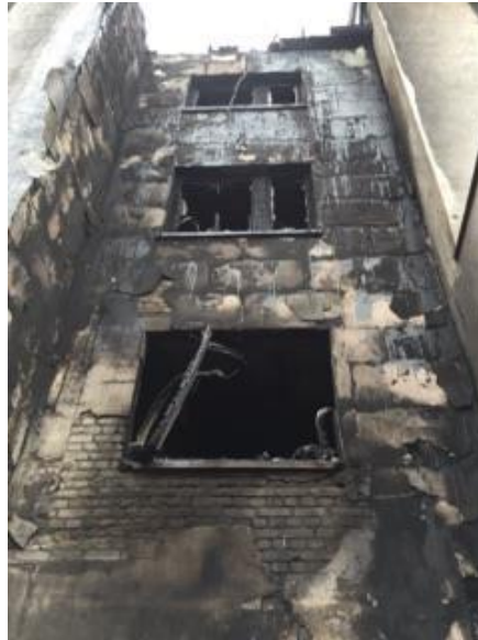
Figure 35 – ETICS Façade fire at Apartment building in Duisburg [75]
