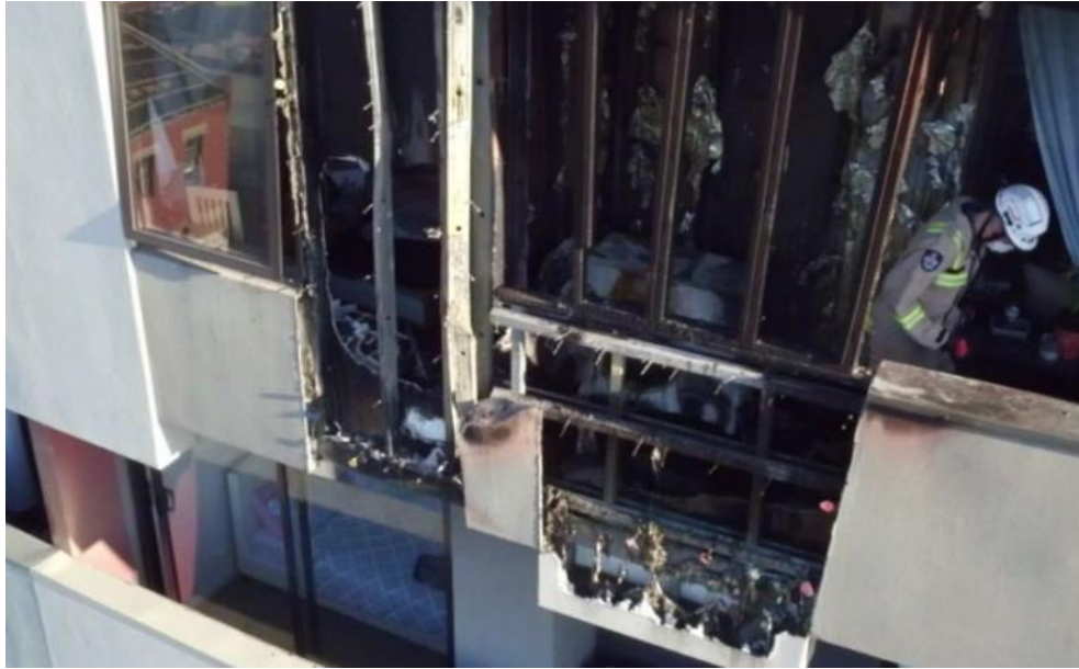
Figure 31 - Photo of Anstey Square Complex after fire spread from one apartment to the next [74]
