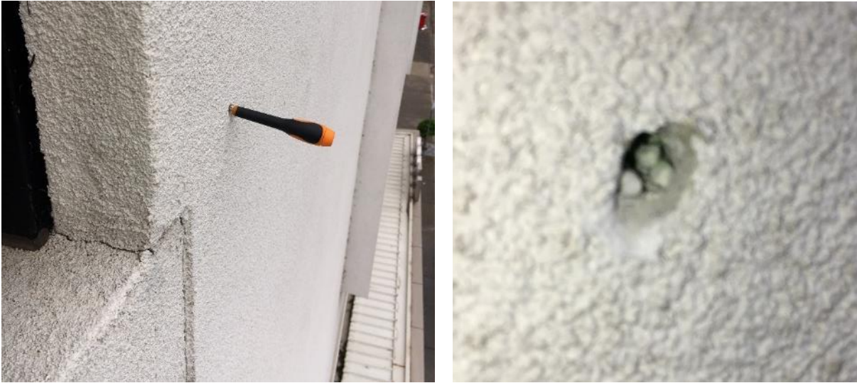
Figure 20. Probe used to penetrate EPS EIFS system render. In this case the render was ~ 5-6 mm thick and felt like compressed cement sheet based on external knocking only and was initially difficult to penetrate with probe. Thinner renders will have a different feel and be easily penetrated. (Photos by CSIRO)
