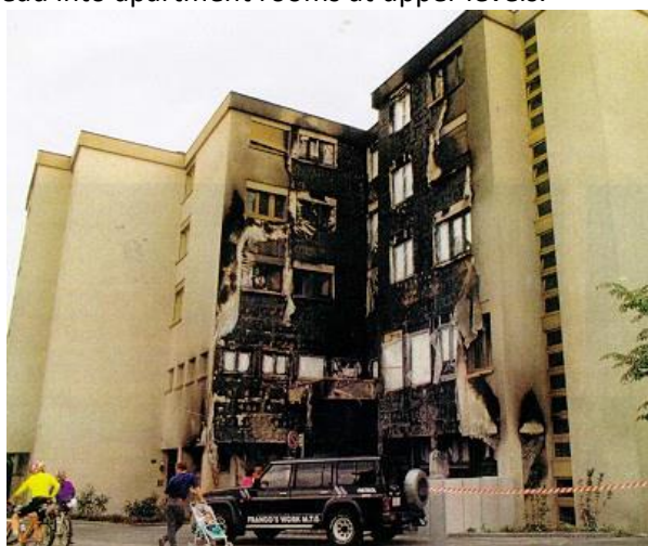
Figure 49 - Munich EIFS fire 1996 [78]
