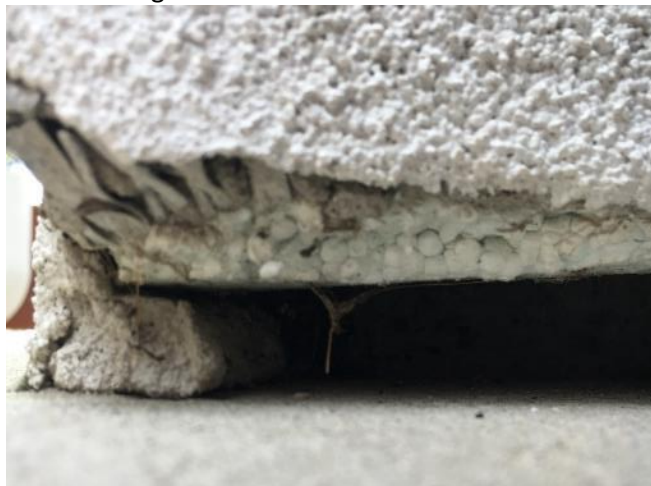
Figure 17. Example of bottom edge of EIFS exposed (photos by CSIRO)
