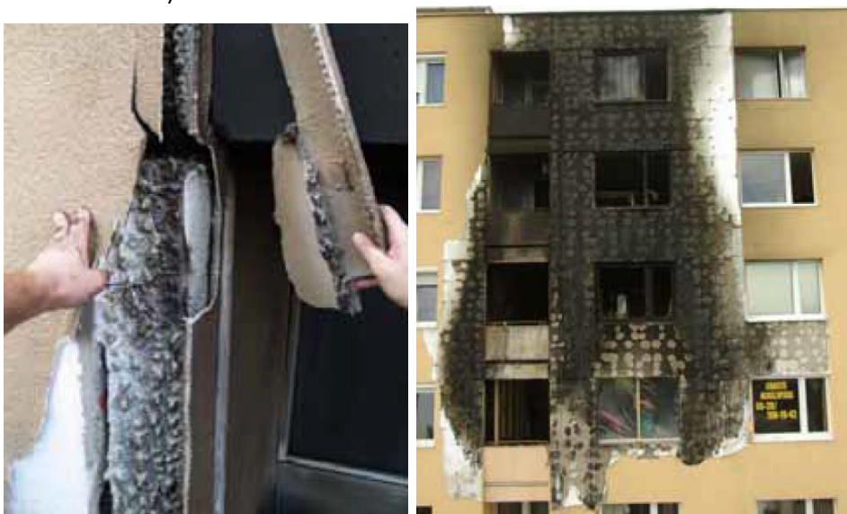
Figure 46 – EIFS fire in Miskolc showing damage to cladding (LHS) and extent of damage to façade (RHS) [81]
