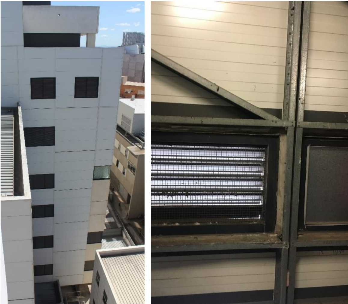
Figure 21. Example of ISP with PIR core as external wall on multi-storey building viewed from exterior and interior within plantroom. (Photos by CSIRO)
