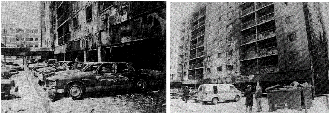
Figure 50 - Damaged cars outside east wall (LHS) and extent of damage to east and north walls (RHS) [82-84]
