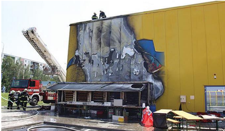
Figure 56 – PIR Insulated Sandwich panel post fire damage on Furniture Retail Warehouse, Slovakia
