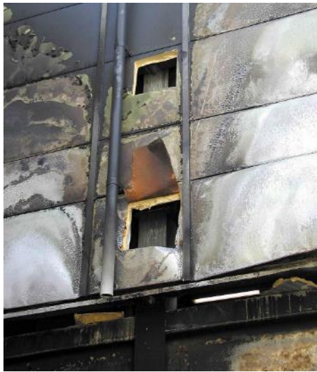
Figure 54 – PIR Insulated sandwich panel post fire on Wharfedale Hospital, UK
