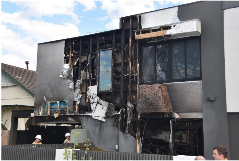
Figure 33 - Post fire damage to street frontage shown on two storey unit (Photos provided by MFB)
