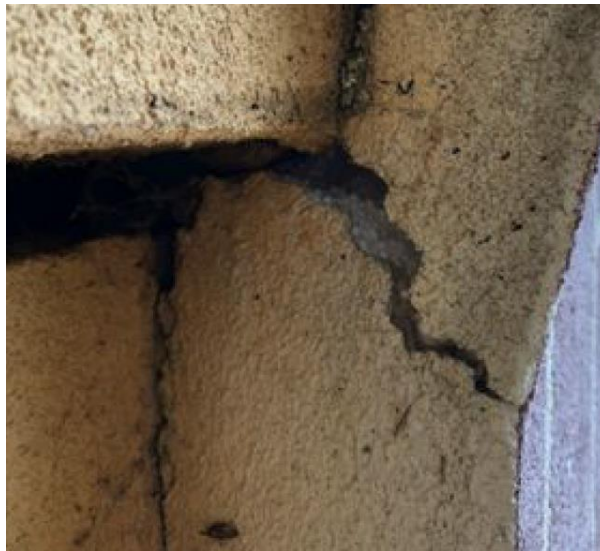
Figure 18. Damage to EIFS system with inappropriately thin render systems and poor maintenance (example photo extracted from ARP building audit report).
