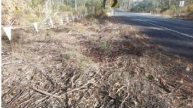
Photo 2: Pyrenees Highway, showing ground cover for fauna habitat (CH 11.115 - CH 11.150 LHS formation widening (fill construction))
