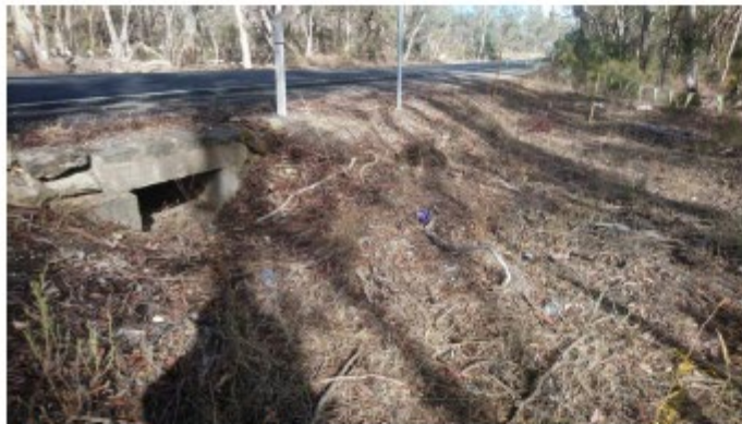
Photo 3: Pyrenees Highway, showing ground cover for fauna habitat (CH 13.610 - CH 13.690 LHS formation widening (fill construction))
