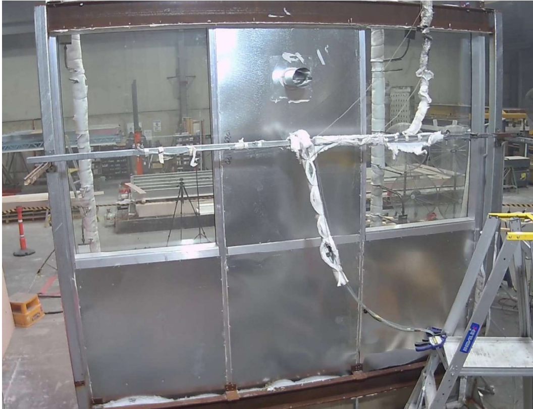
Figure 44 The unexposed side of the specimen at the end of test.
