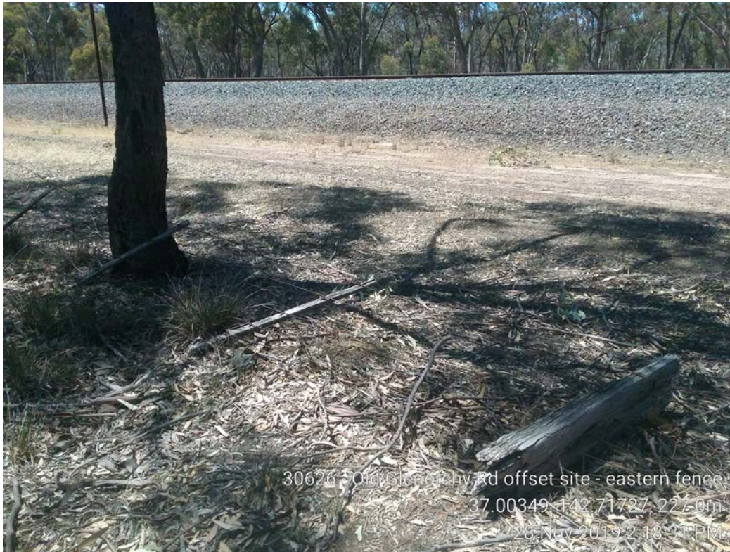
Plate 3 Fence condition along the eastern boundary with the rail reserve
