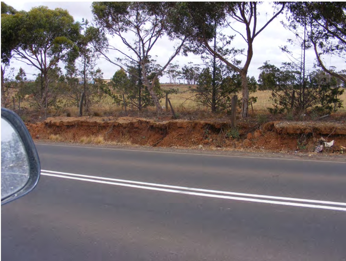
Erosion on Sinclairs Rd north of Kororoit Ck
