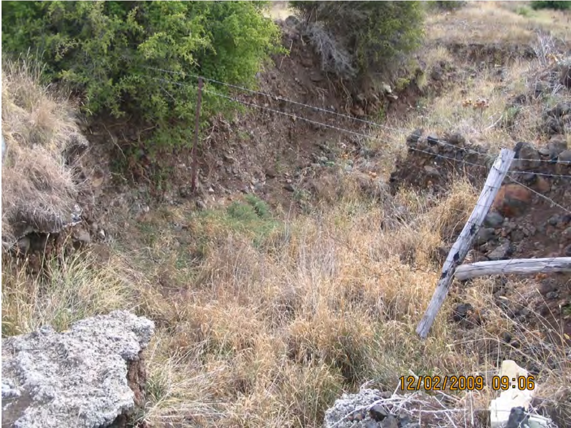
Morefiled Ct creek bed adjacent to culvert Showing potentially high water flow at times
