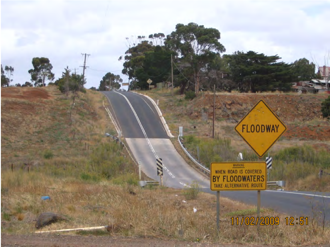
Kororoit Ck on Sinclairs Rd Showing deep creek cutting
