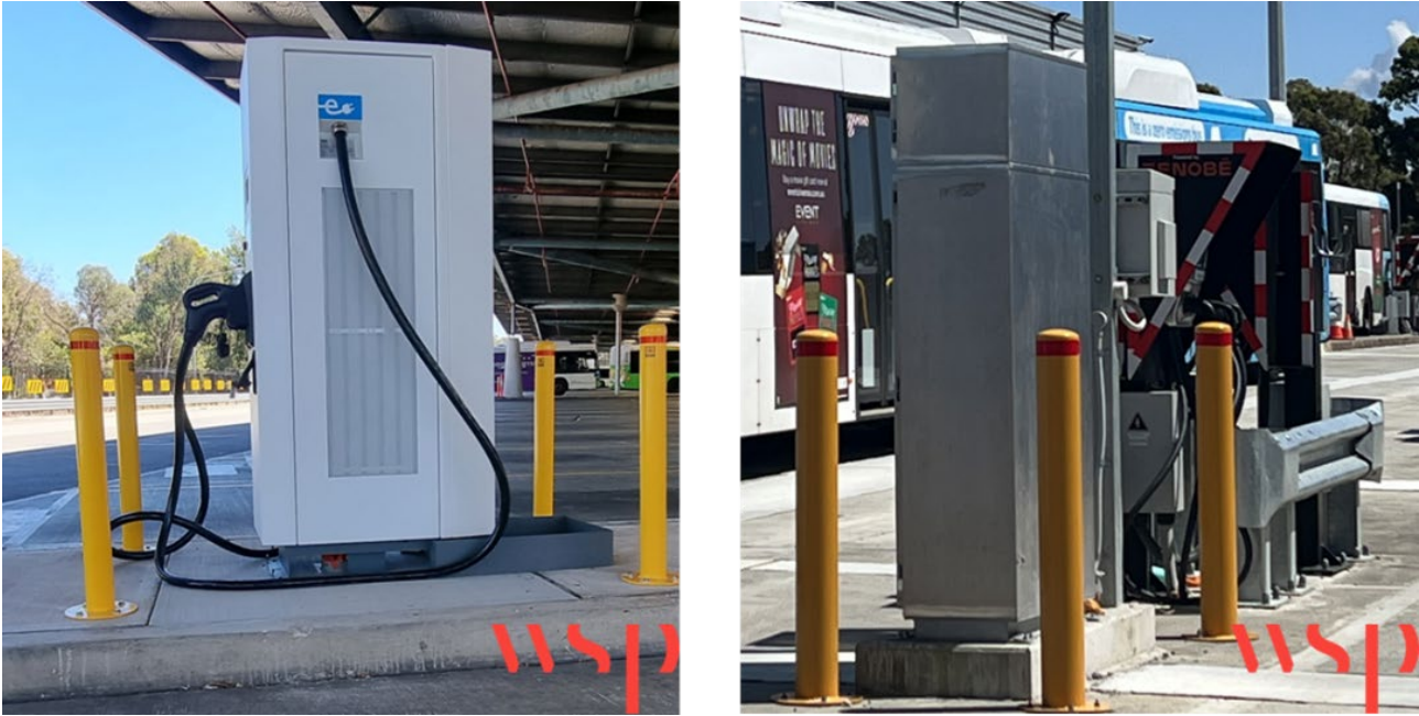
Figure 2.7 Protection of chargers and electrical infrastructure using bollards, kerbs and guardrail. Chargers can be integrated units (left), or consist of a cabinet and dispenser (right)
