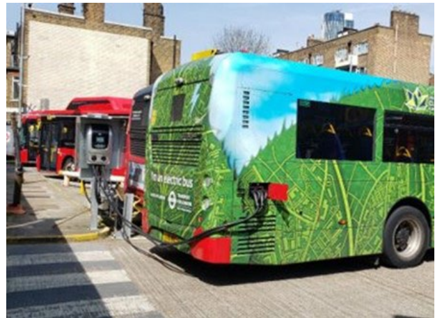
Figure 1.12 Cable wraps around bus as socket and charger are not aligned. Potential for damage to cable due to tension, and tripping hazard in depot
