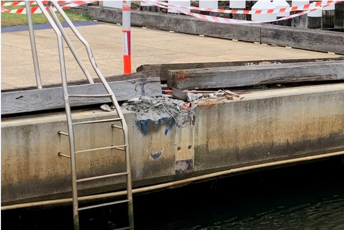
Figure 3: Impact damage to Yanonung Quay wharf
