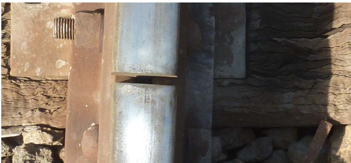
Figure 4: Typical expansion gap in jointed rail
