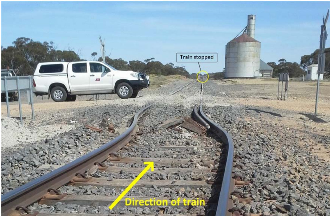
Figure 2: Laterally displaced track just prior to the Janiels Road level crossing, looking in the train's direction of travel.
