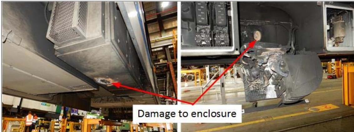
Figure 6 Line Breaker and enclosure damage
