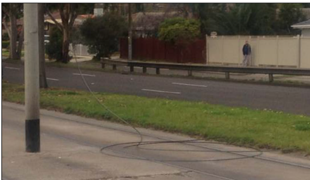
Figure 1: Traction contact wire lying on the tram tracks
