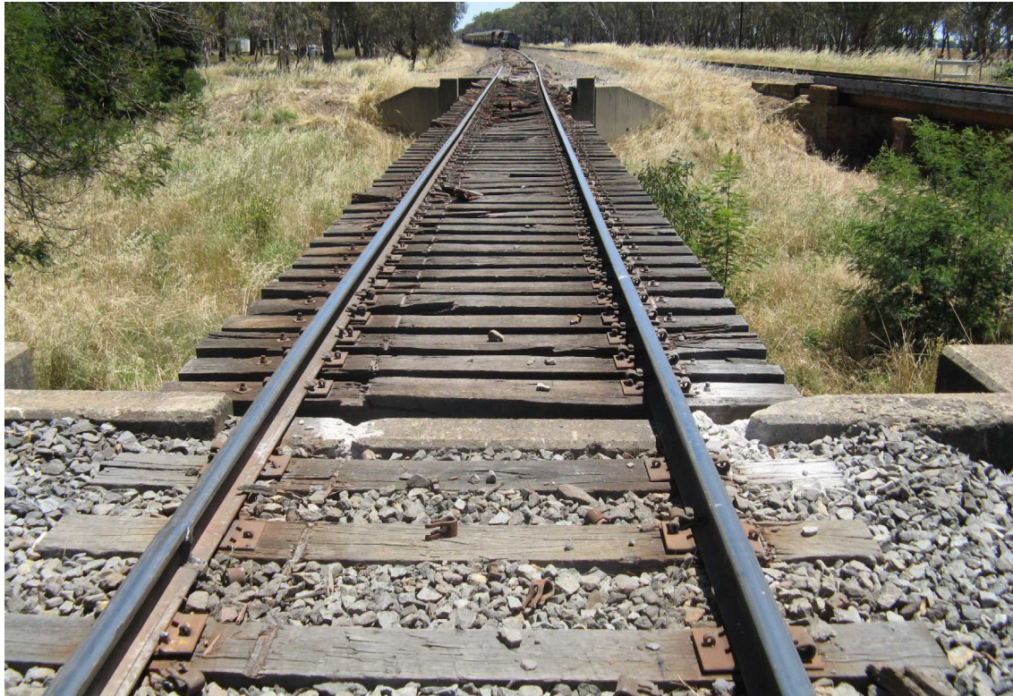
Figure 15 – Damage to the approach end of the railway bridge
