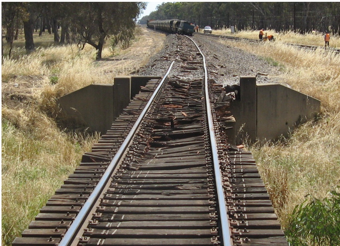
Figure 16 – Damage to the departure end of the railway bridge
