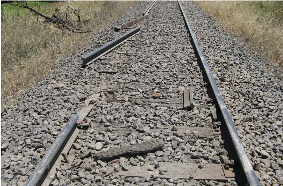
Figure 14 – First rail fracture, about 376 metres after the Down Street level crossing
