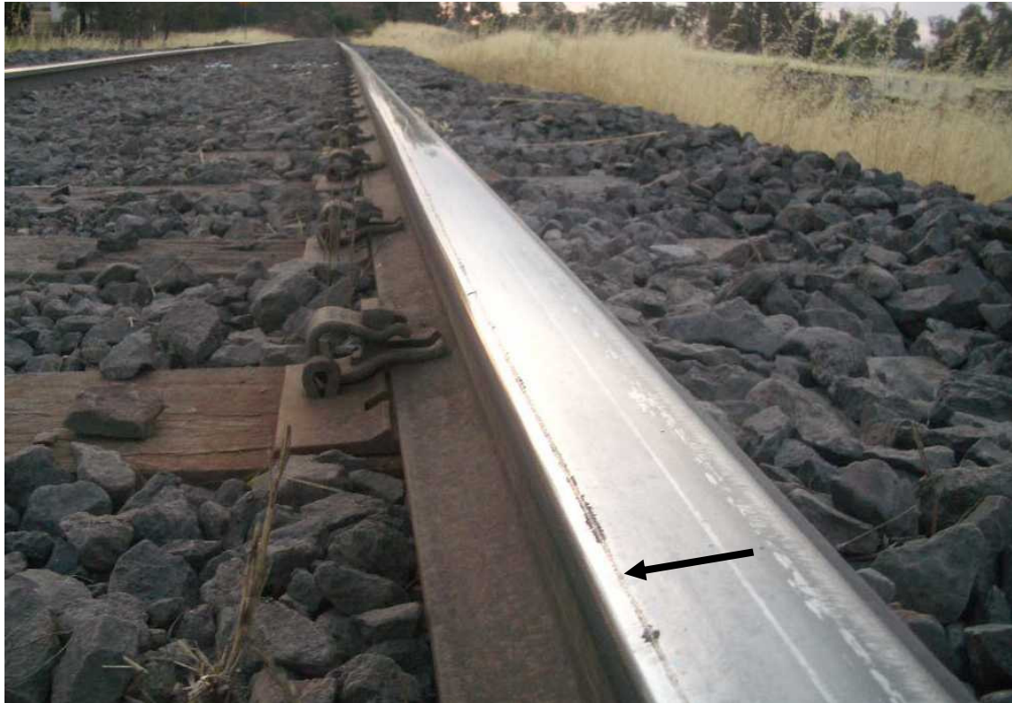
Figure 11 – Flange mark on right-hand rail head extending about 10 metres to the point of drop-off
