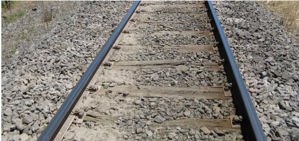
Figure 8 – Ballast condition on Melbourne side of Down Street level crossing, looking south
