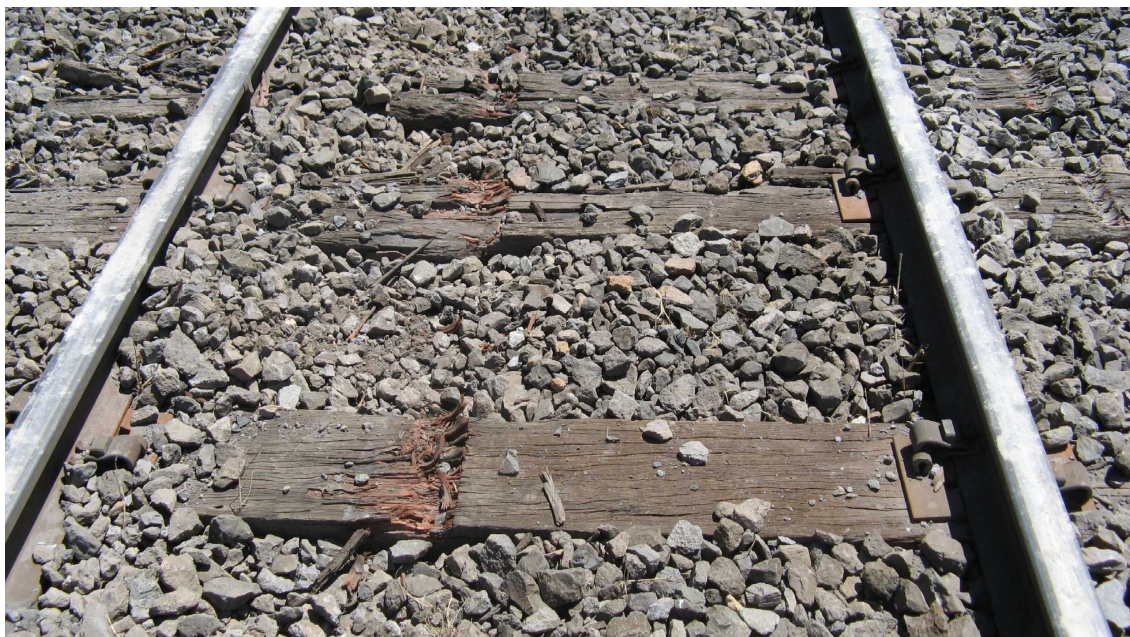
Figure 12 – Typical wheel marks after initial derailment and prior to the first rail fracture
